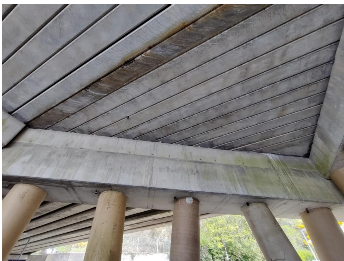
Plate 7.11 Gaps in soffit of the R448 elevated roadway which could potentially be used by roosting bats.
